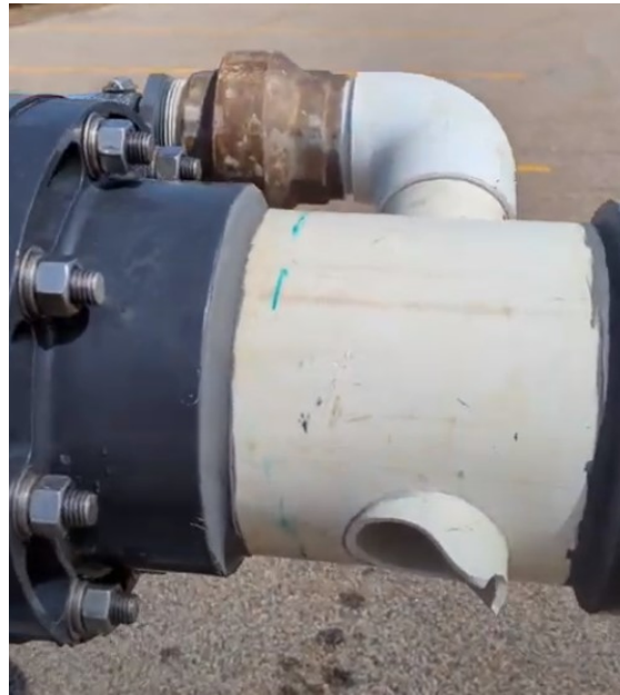
Figure 7.1: Damage incurred to wave pump section's elbow and inlet check valve due to interactions with rocky shore.
