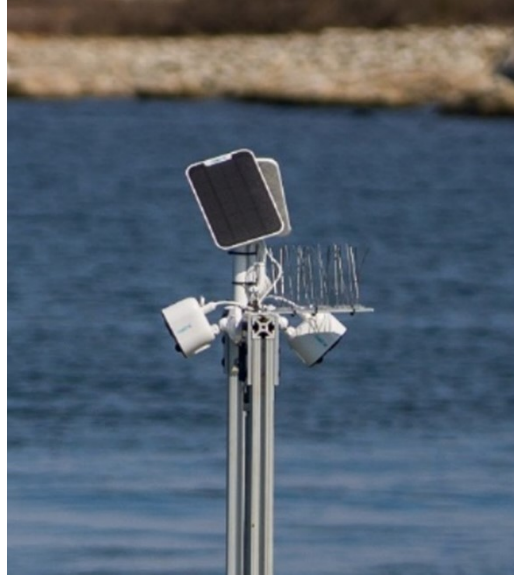
Figure 6.11: Motion triggered video cameras, solar panels, and lidar target installed onto float gantry.
