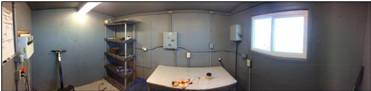
Figure 14: Instrumentation Shed - inside
