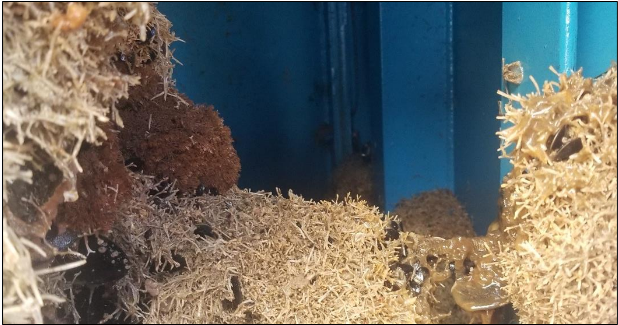
Figure 34: Growth of algae inside entrapped water chamber.
