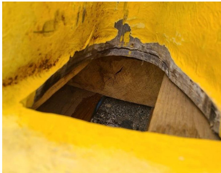
Figure 52 - Cracks at the bottom of the heave plate float.
